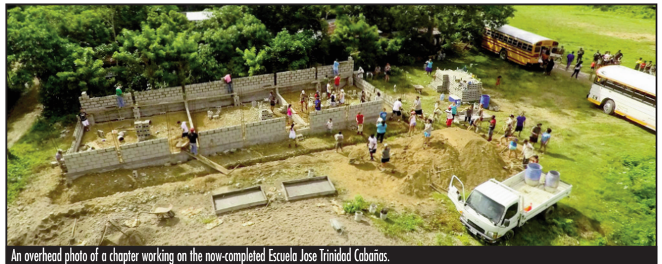
An overhead photo of a chapter working on the now-completed Escuela Jose Trinidad Cabañas.
